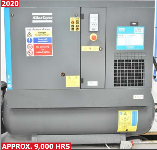
APPROX. 9,000 HRS ATLAS COPCO G11FF 15 HP rotary screw air compressor
