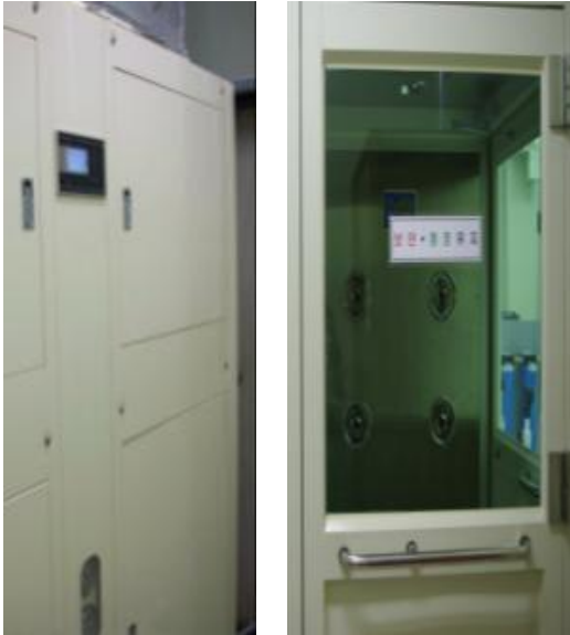
-Environment Controller -Air Shower Rm.
