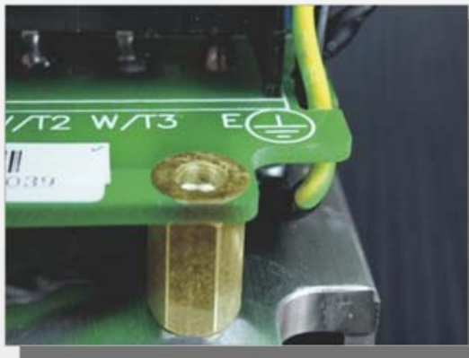
Board to ground
