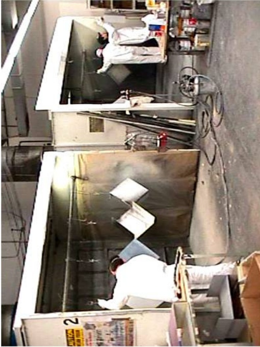
Paint Spray Booths
