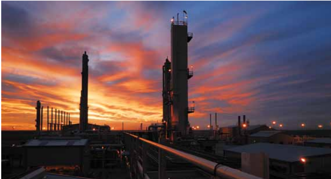
Nitrogen rejection unit
