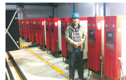
Fujian Zhanpin power plant
