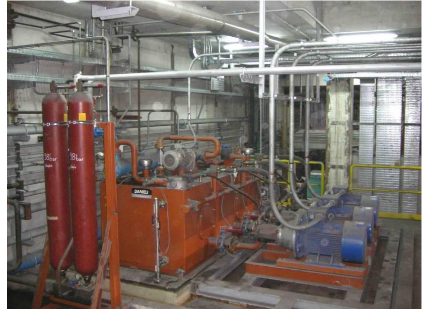
Mill Hydraulic Control Room
