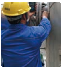
500°C Steam Pipe
