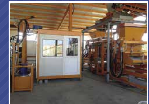
Control cabin with PC and cables of connection of units and assemblies
