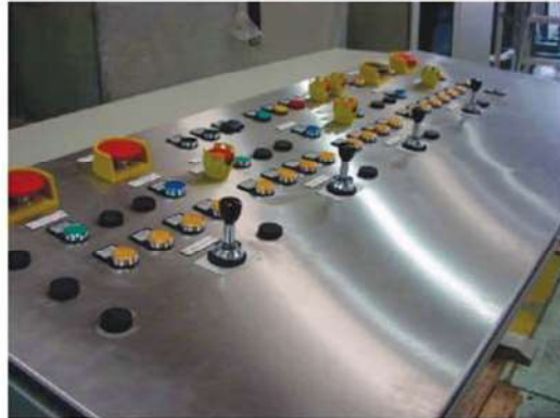
Main Control Pulpit
