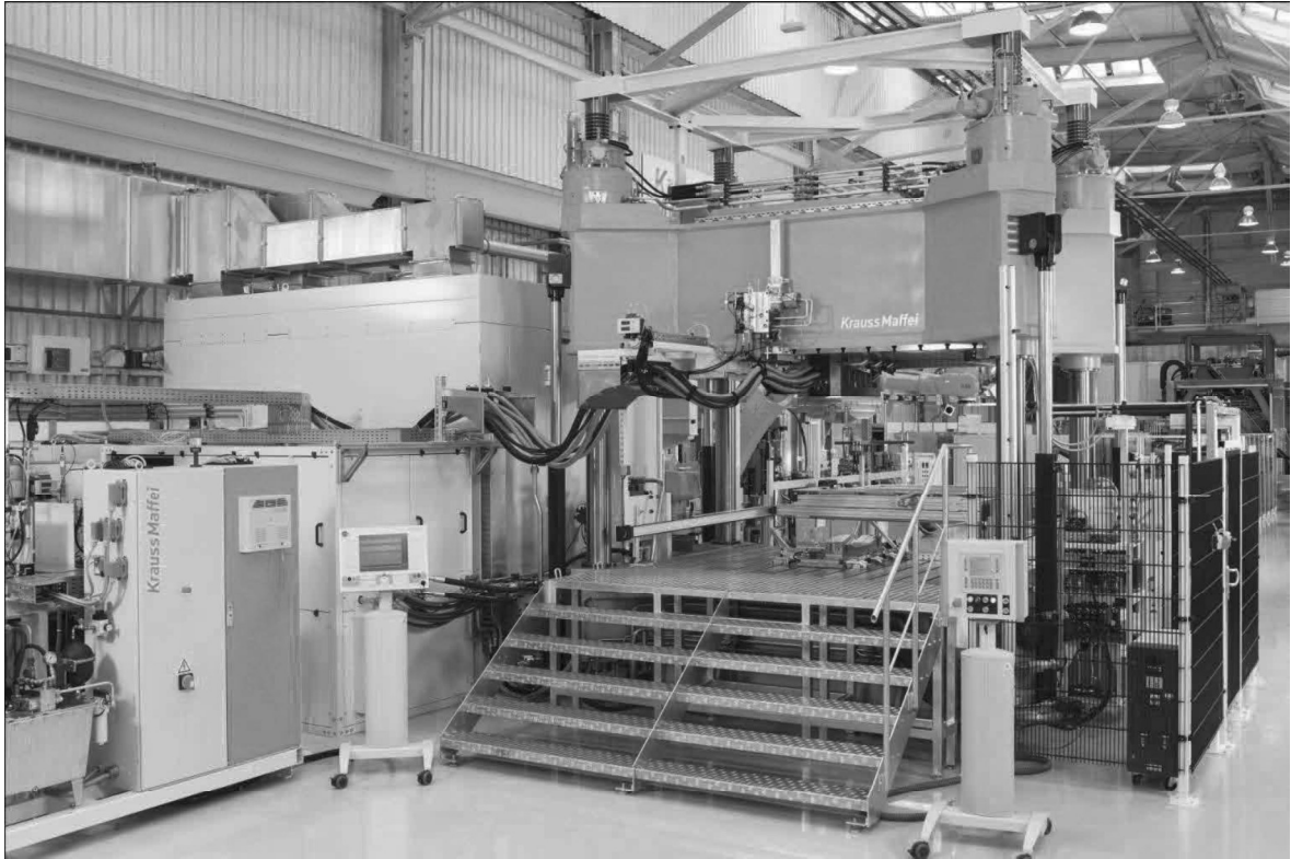
SFT MX600T Mould Carrier Installed in the Composites Demonstration Facility, Munich, Germany
